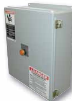
Multiple-Operator Junction Box
