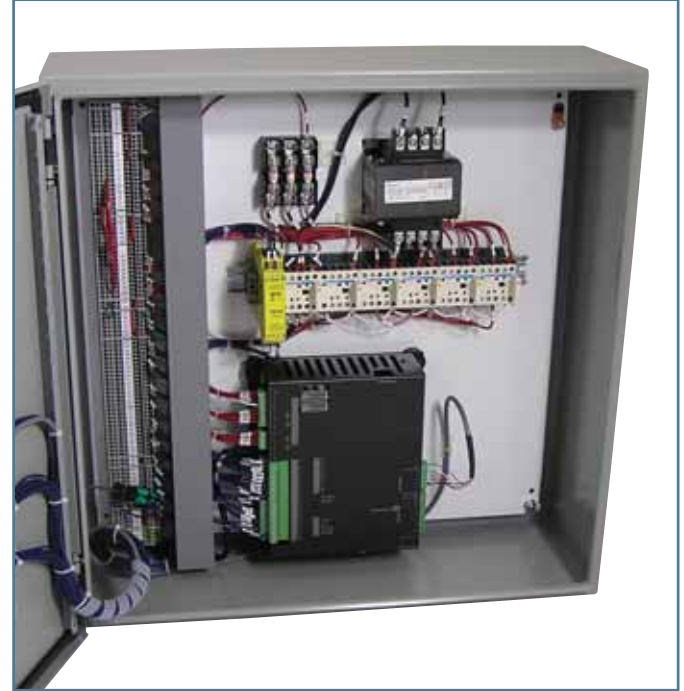
Standard Control Box—Inside View
